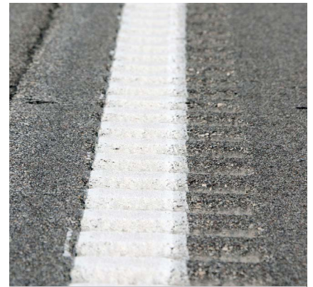
Example of an edge line rumble stripe.
