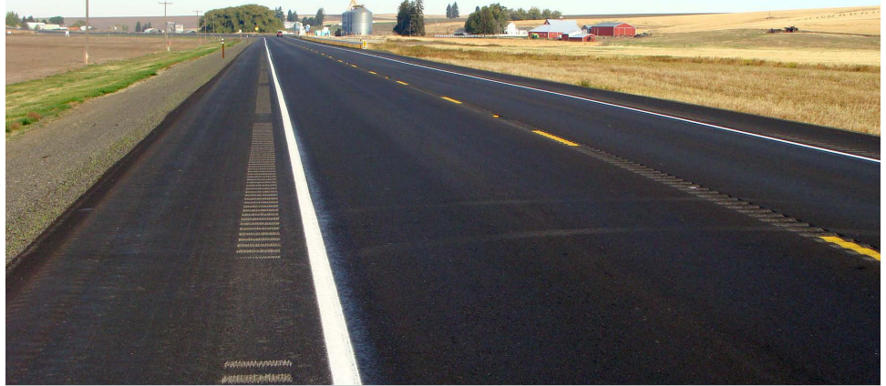
Shoulder rumble strips and center line rumble strips are installed on this roadway.
